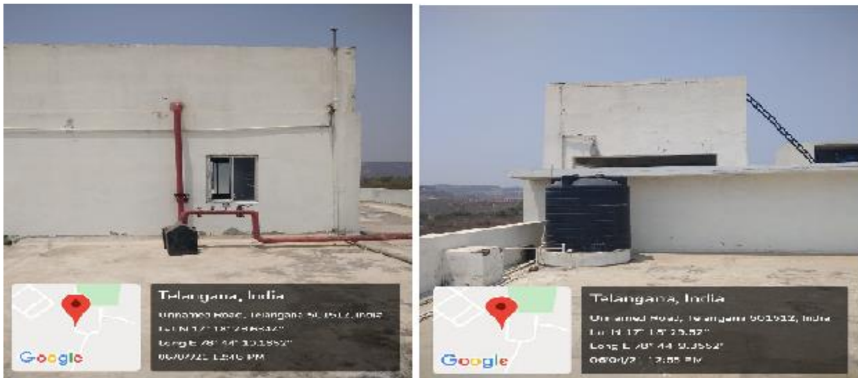
OVER HEAD WATER TANKS
