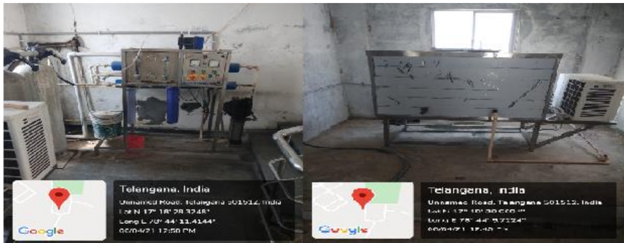
RO WATER SYSTEM
