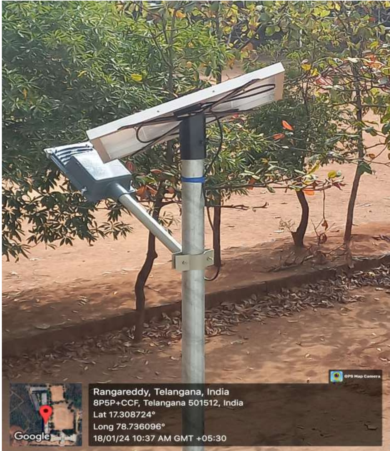
Sensor-Based street lights in Campus.
