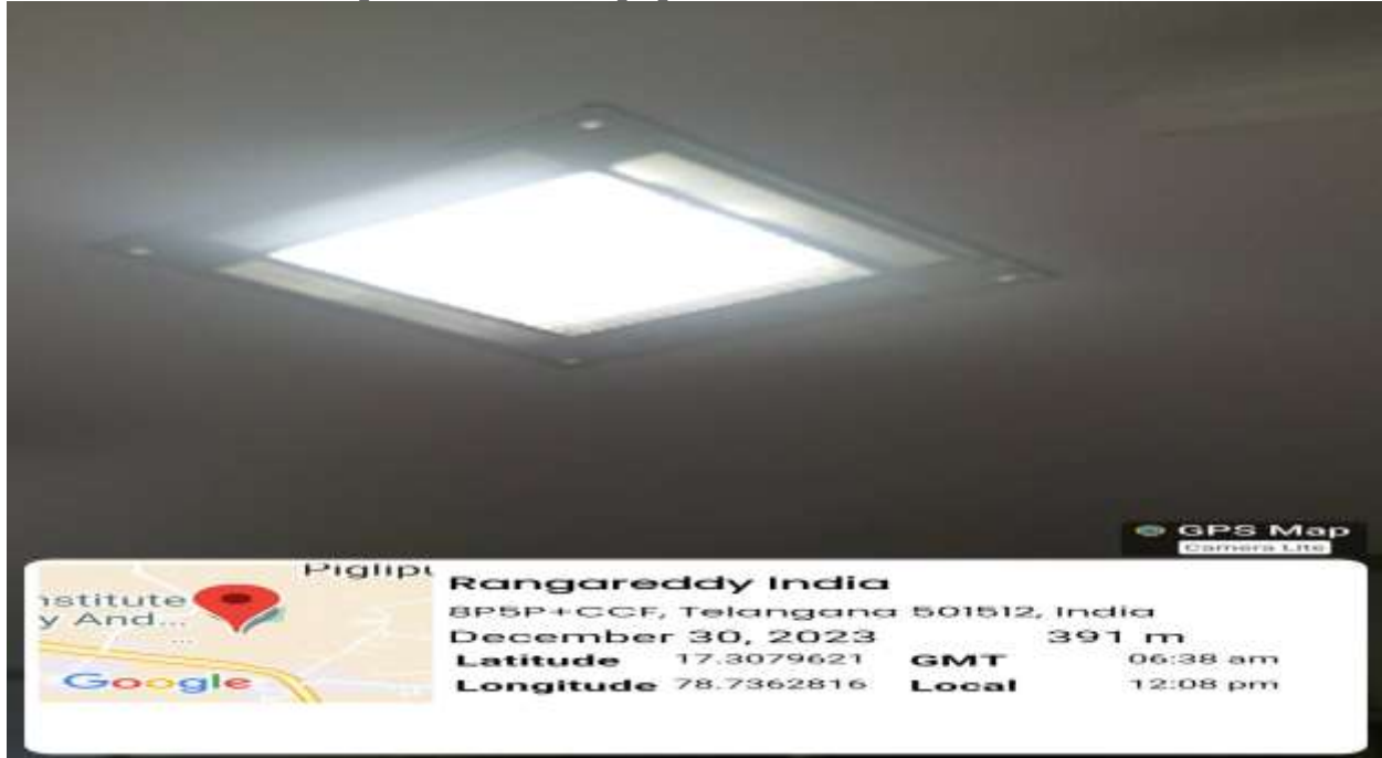
Usage of LED bulbs in LAB
