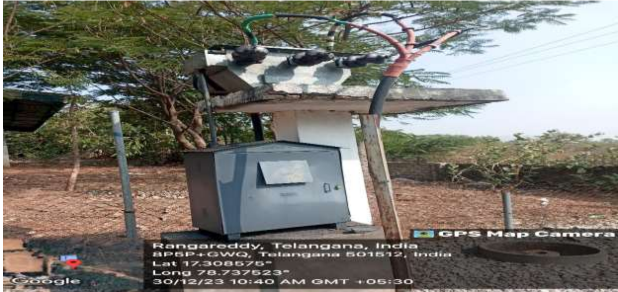
Wheeling to GRID connection.
