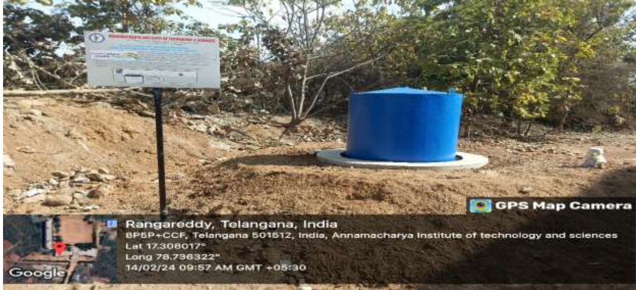
Bio Gas plant at college
