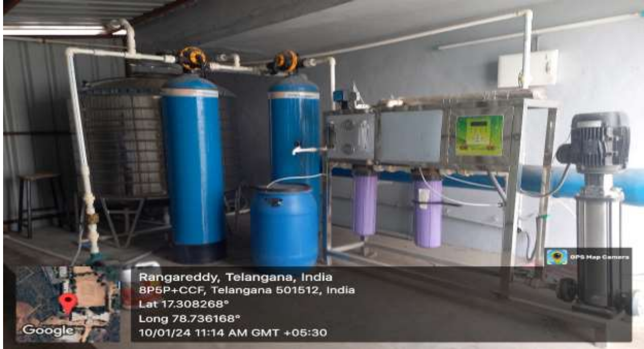
RO water plant
