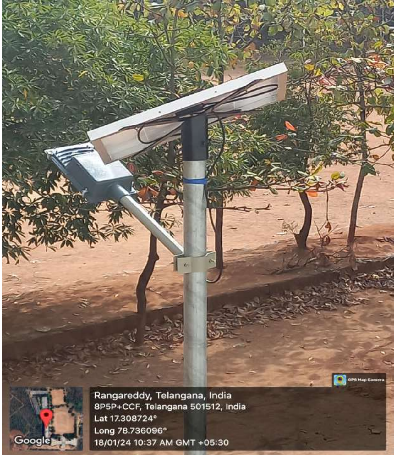
Sensor-Based street lights in Campus.
