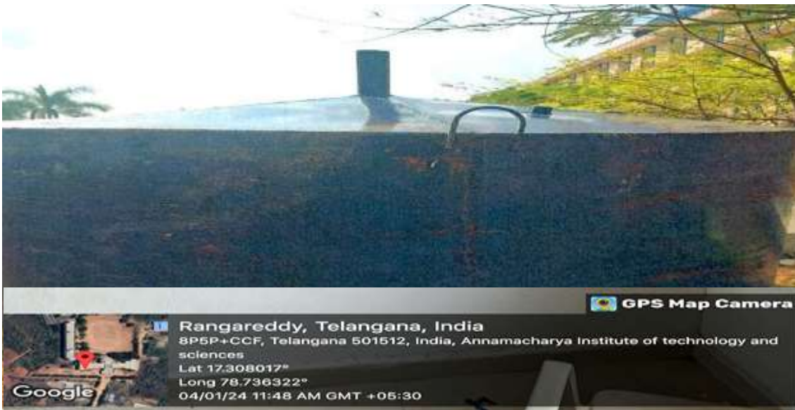
Bio Gas plant at college
