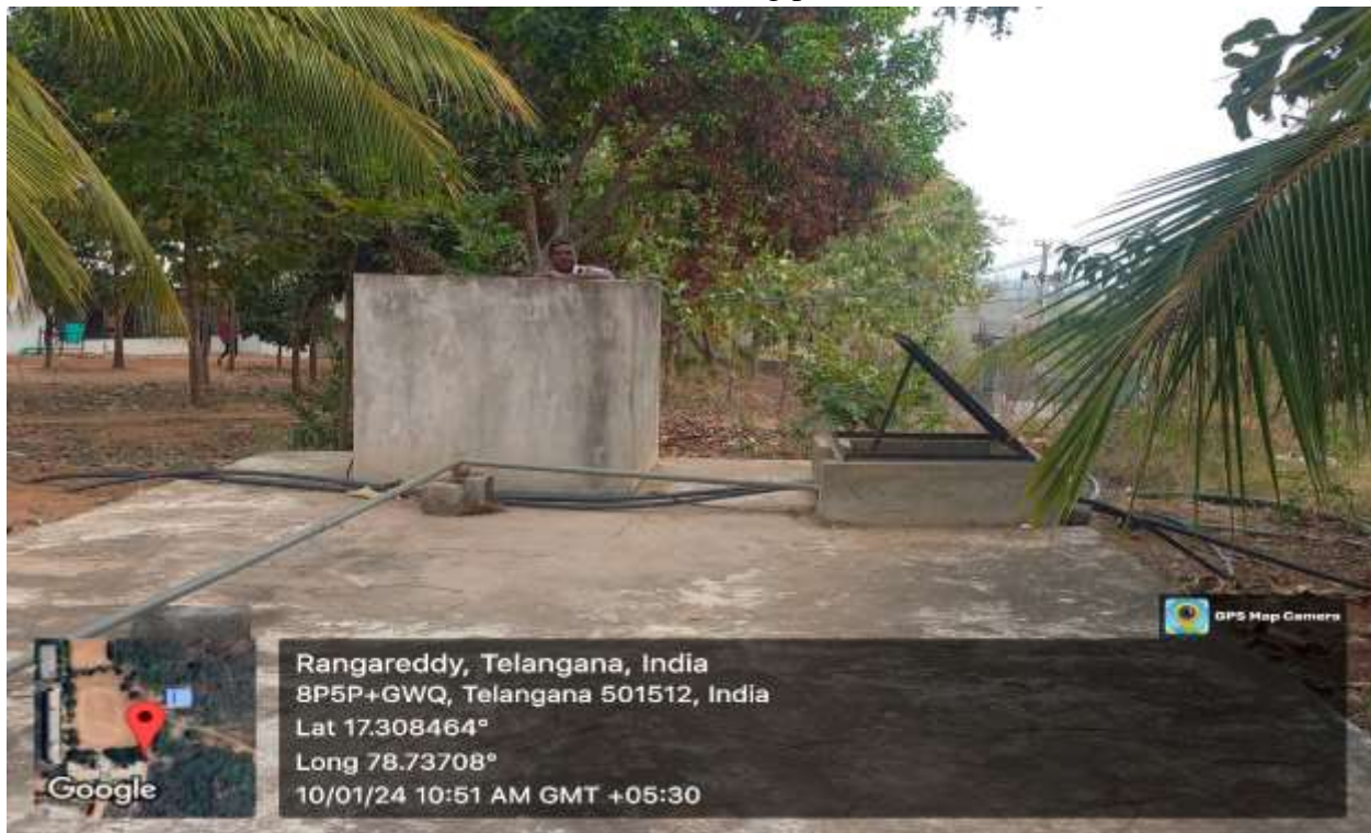
Bore well recharge pit
