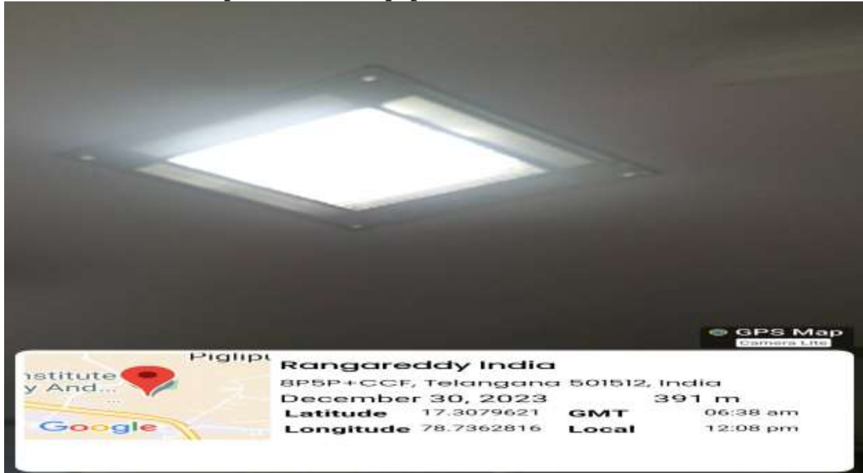
Usage of LED bulbs in LAB
