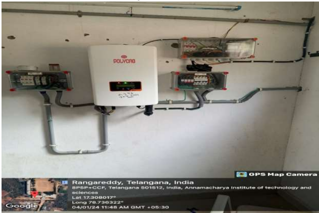
Wheeling to GRID arrangement with display of Metering.
