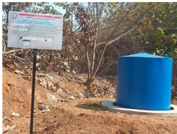
Bio Gas Plant
