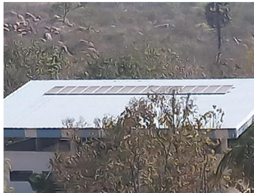
Solar Power Plant
