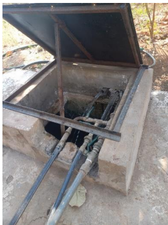
Rainwater harvesting tank
