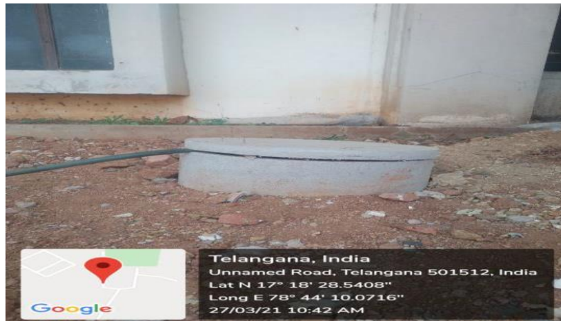
Rain Water Harvesting Tank
