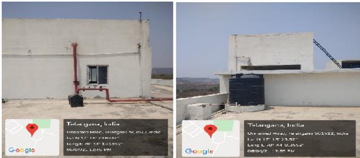
OVER HEAD WATER TANKS
